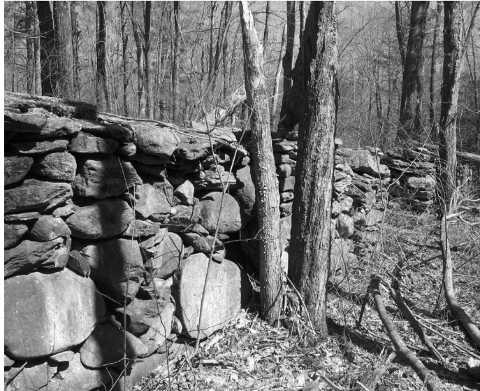
The 'Noble Wall' structure today, originally built as a kitchen garden for Timothy Ruggles' proposed homestead Coxhall
