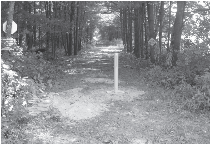
Newly installed bollard at the New Braintree Train Station
